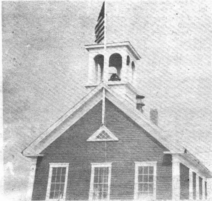
The newly renovated cupola is back at home on the Whitneyville Town Library. (Clancy Photo)
